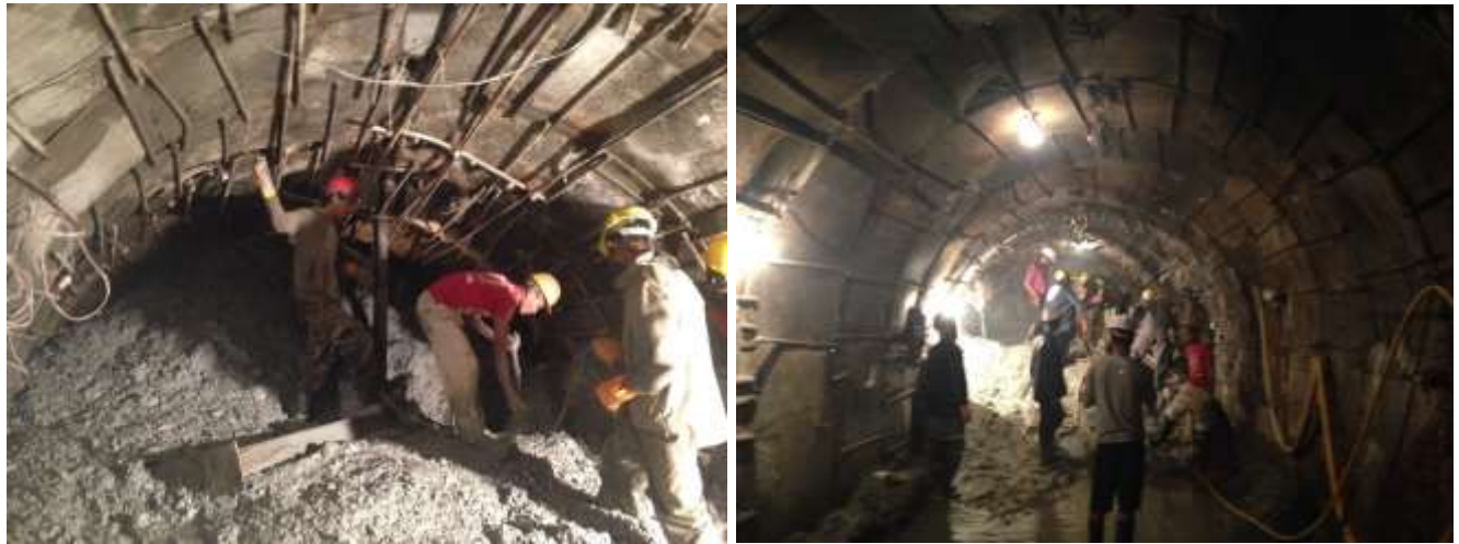
Poor Rock Condition encountered at Tunnel face @ CH 0+200 m.
