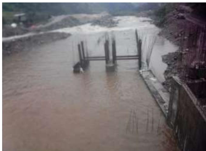
Flood at Headworks
